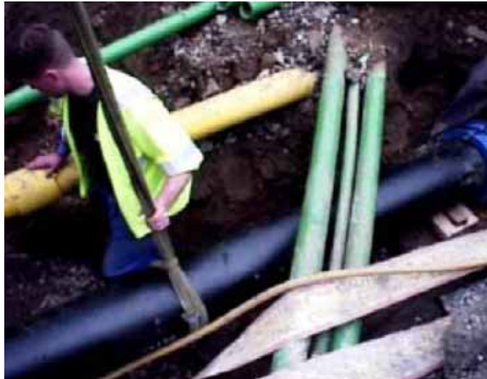
Figure 1: A typical tangle of pipes and cables under our city streets that can result in expensive third party damage
